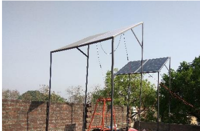
Solar PV system installed at the representative's location
